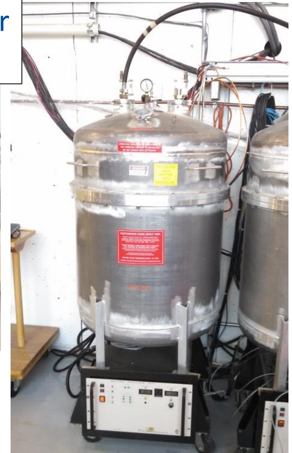
170kV Power Supply
