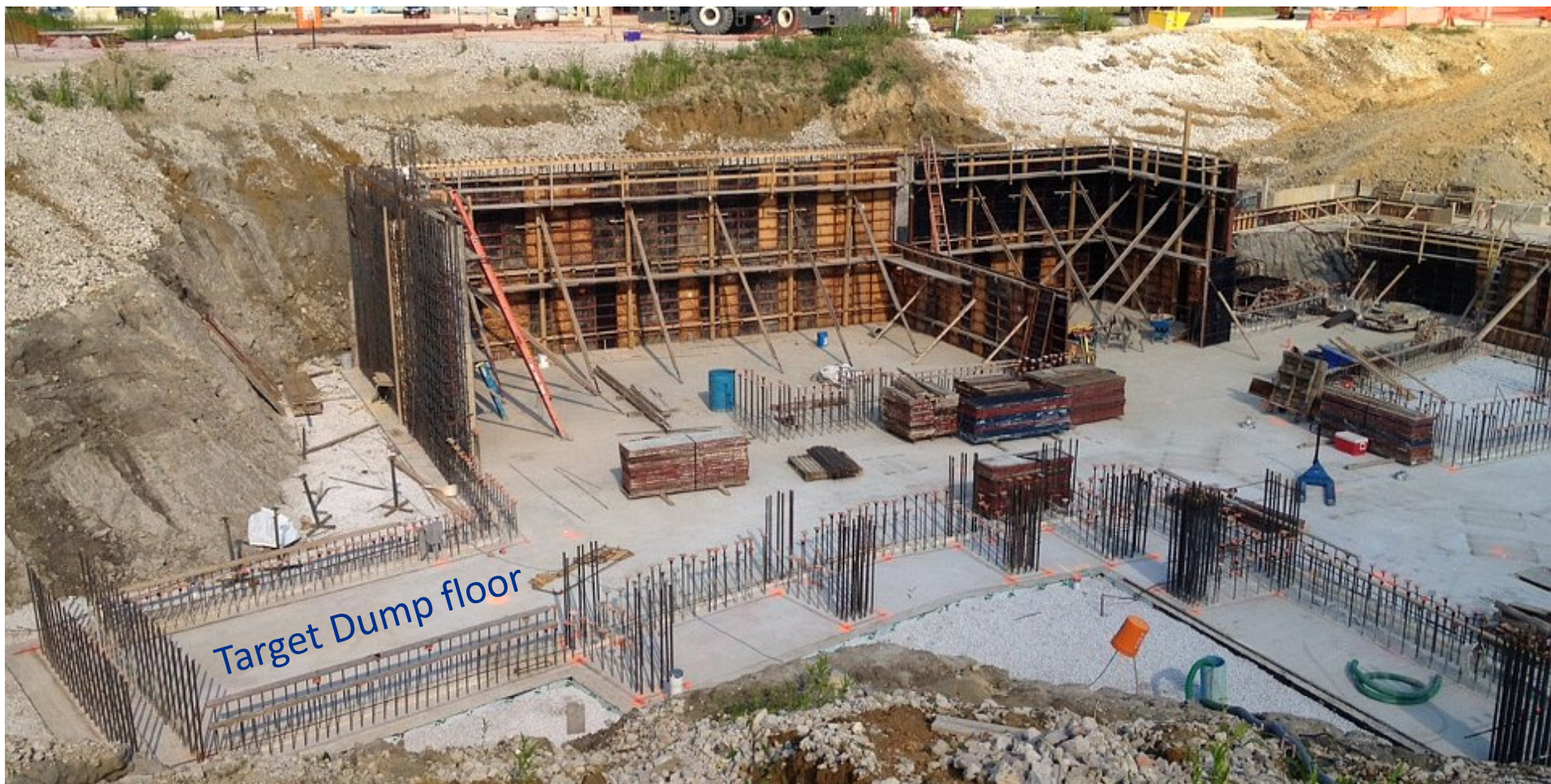
Framing the walls in the proton target station area of the Mu2e building
