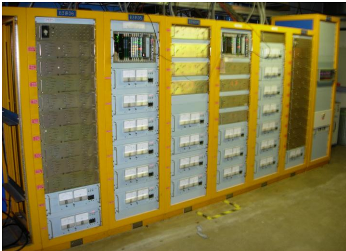
Vacuum Controls at AP30 service building will be repurposed
