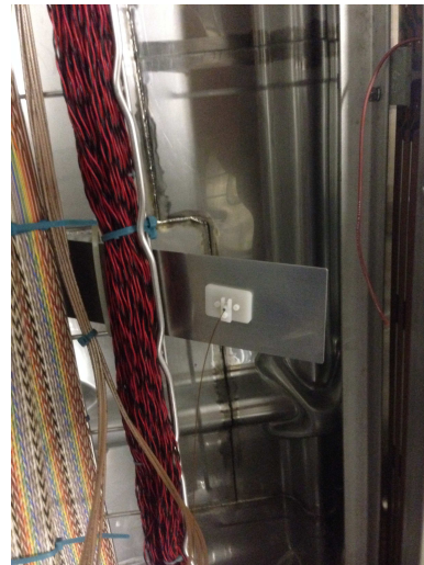
Figure 1: Flasher installed on the leftside of the APAs to flash light behind the APAs (unsuccessful due to optical fiber break).
