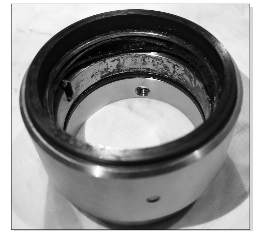
Sliding ring of an oil pump, despite moderate fluid temperatures local overheating lead to damage and fail
