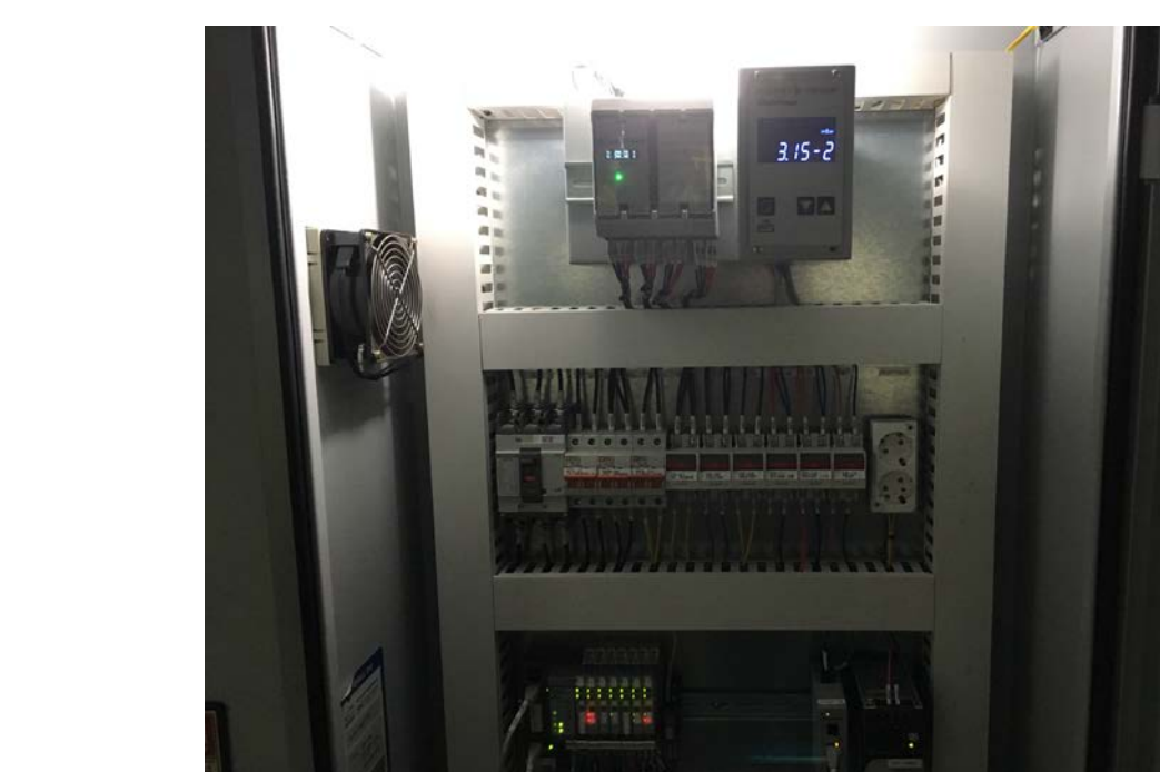
Valve box control panel
