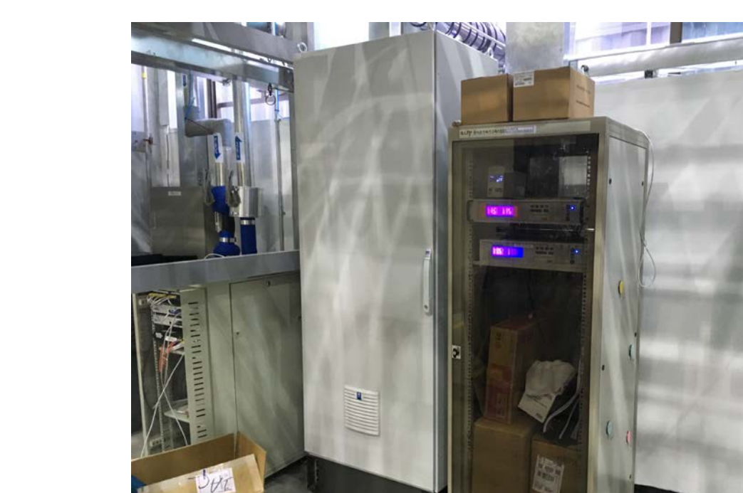
Distribution Box control panel
