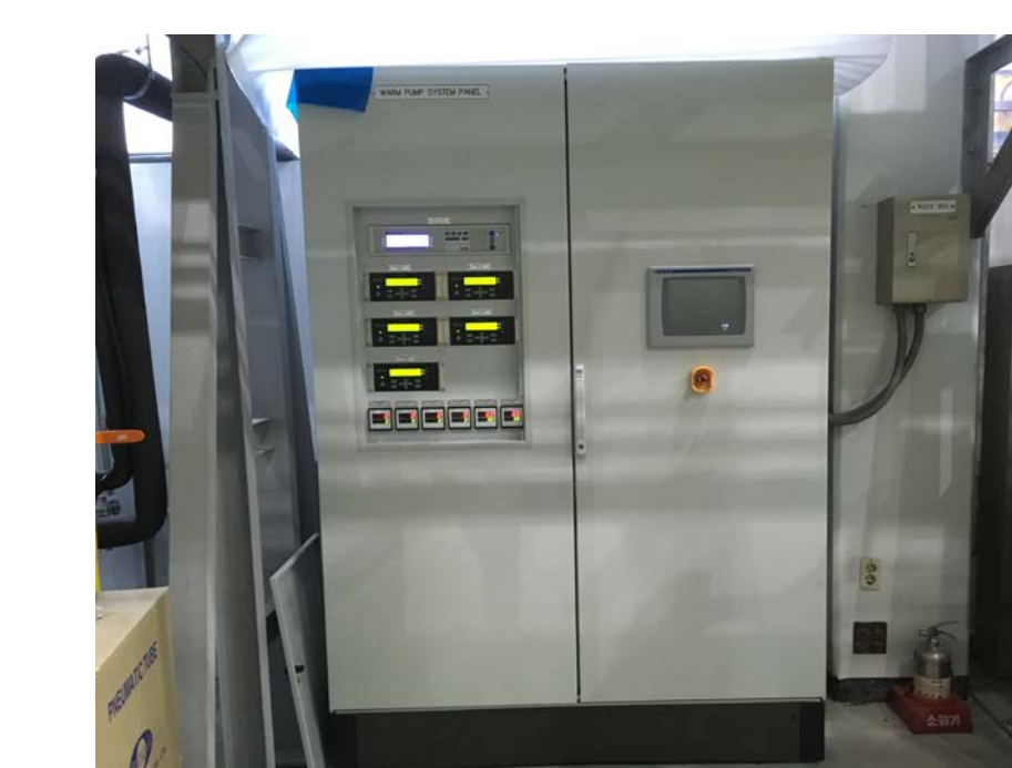
Main control panel
