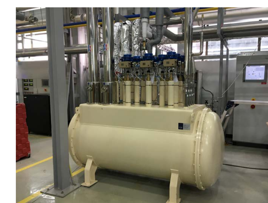
Distribution box and helium transfer lines
