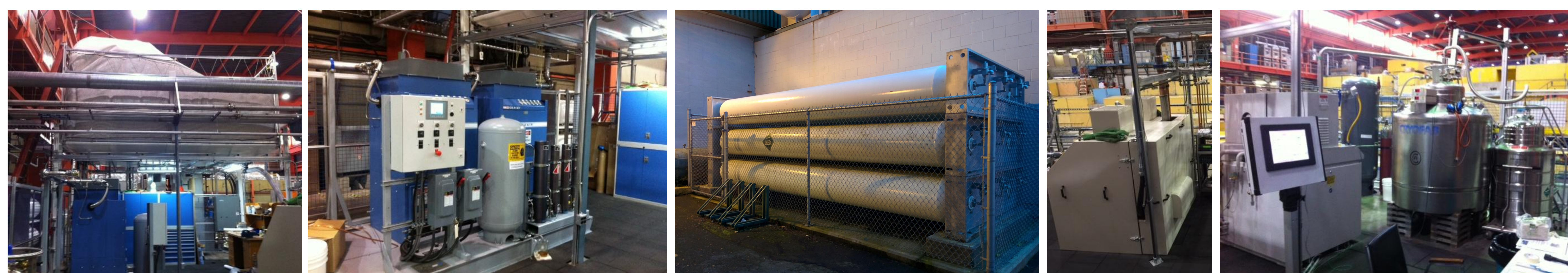
Helium storage bag, high-pressure compressors, high-pressure cylinders, Linde 1610 compressor and liquefier
