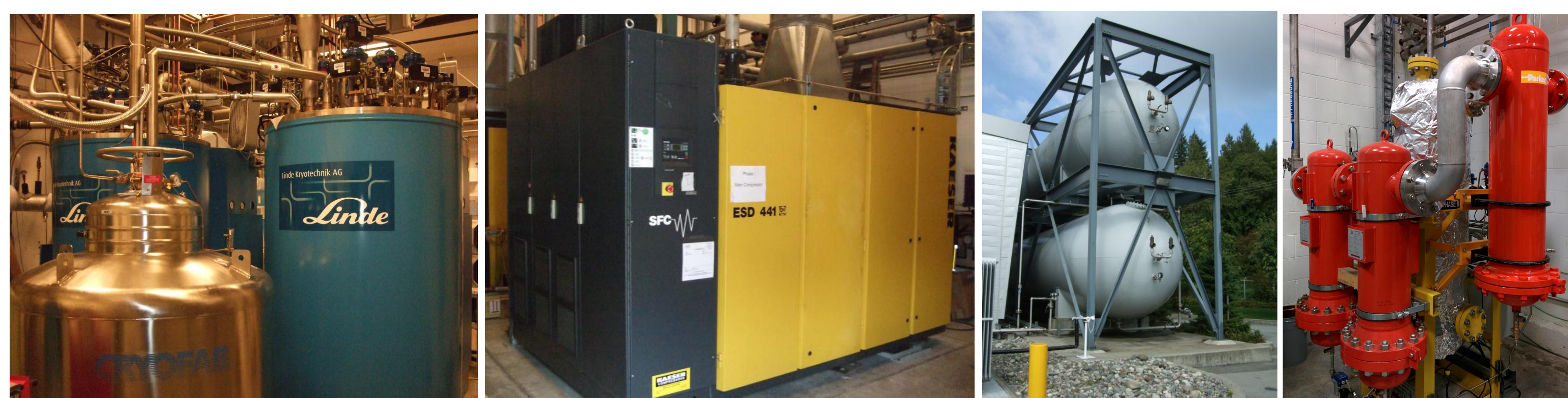
Linde TCF50 helium refrigerator, main compressor, storage tanks, upgraded ORS
