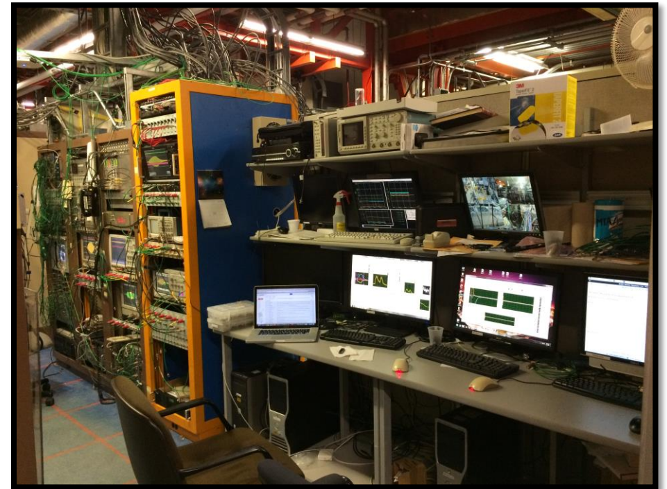
Run control station at the linac gallery
