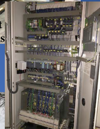
Tracking Control Cabinet
