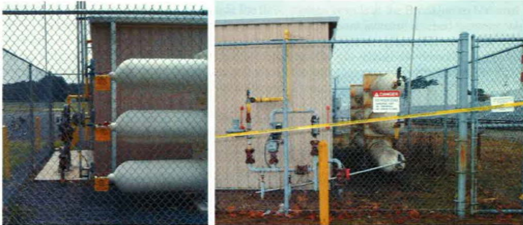
A View of the High Pressure Natural Gas Storage Vessels with the Failed Relief System Before (left) and Aft
