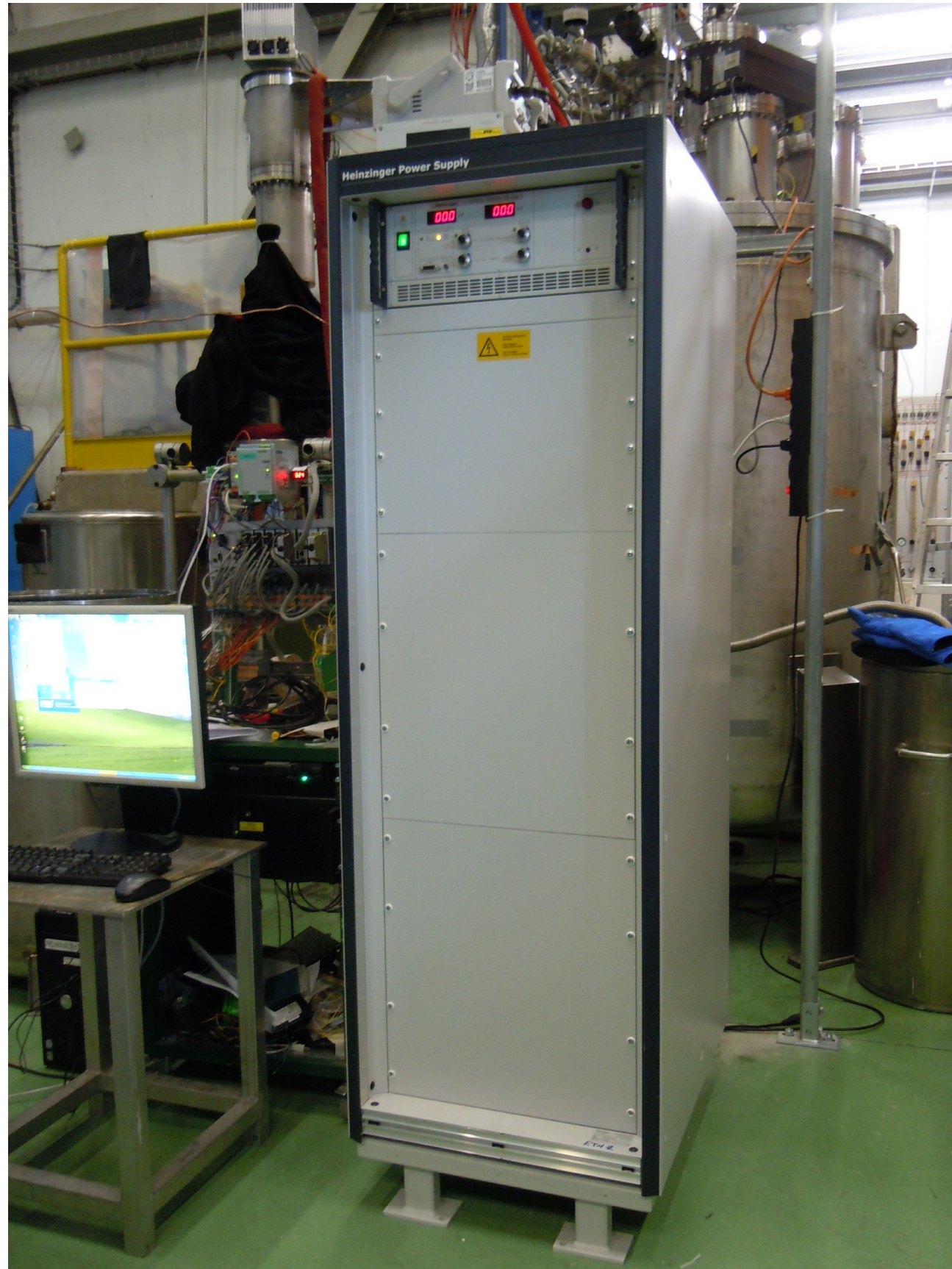
Heinzinger 300 kV Power supply
