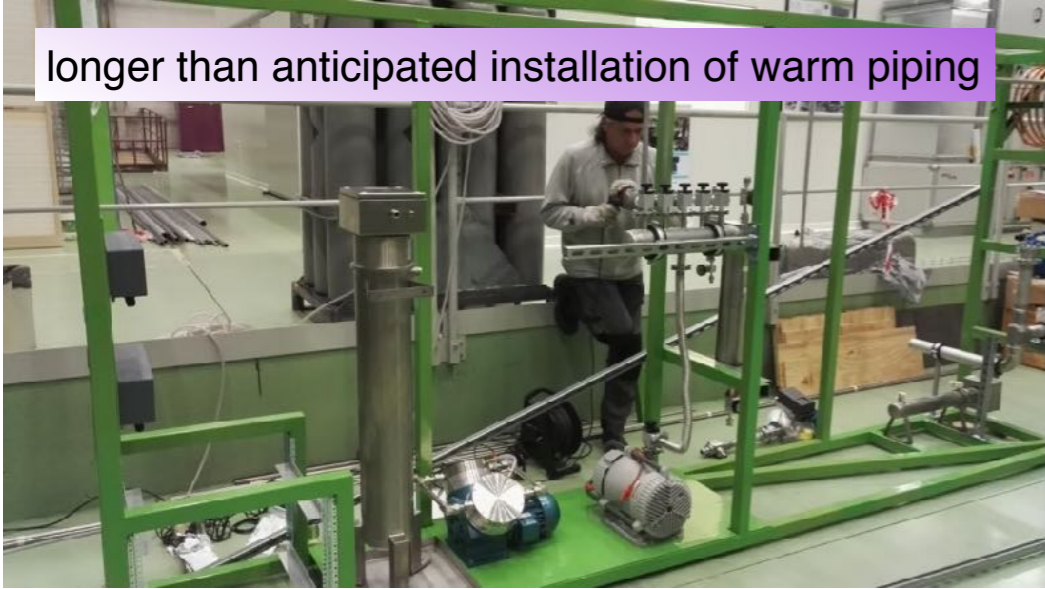
broken bellow at the middle of pump tower
