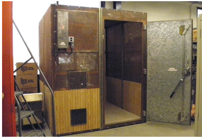
Figure 18: RF copper screen shielded room.
