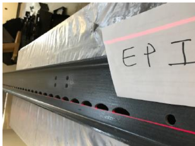
Figure 3: Checking the alignment of the pattern of aluminum profiles slots with a laser level
