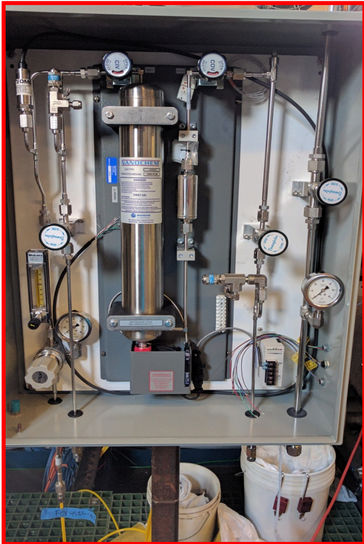
Nitrogen Gas Control Panel
