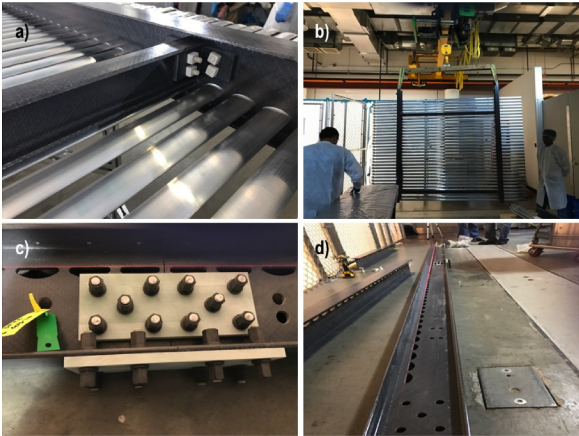
Figure 3.2: (a) A photo of a connection between 6” and 3” I-beams with an L-bracket, inserts (unseen since they are in the screw holes), threaded rods and plastic nuts. (b) A photo of a completed sub-module hung from a crane (c) a photo of an inter-module connection using flat FRP plates, inserts (unseen), threaded rods and hex nuts (d) a 6m long connection of three 6” I-beams. The laser level beam line shows an excellent alignment of the profile slots across the three different beams.
