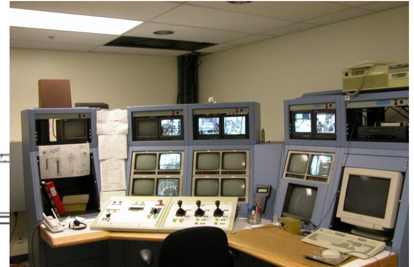
Remote crane control room
