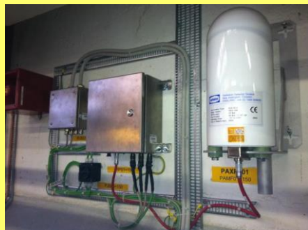
Area radiation monitoring
