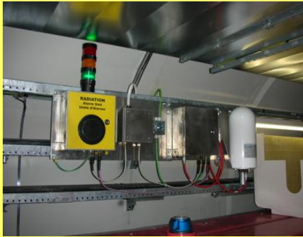
Area radiation monitoring With Alarm unit
