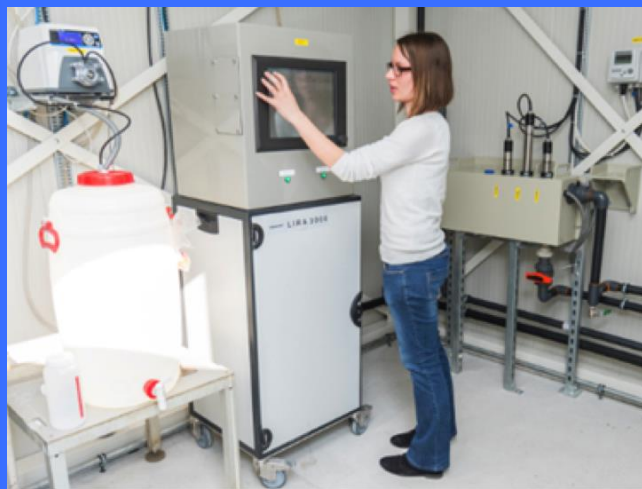
Water Monitoring station
