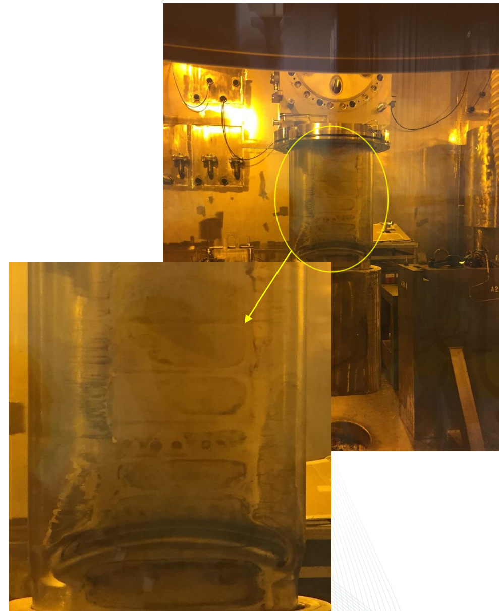
Water Stains Visible on Target Water Shroud
