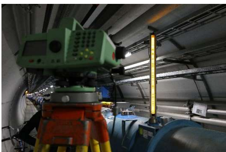
Figure 1: Digital levelling system in LHC.
