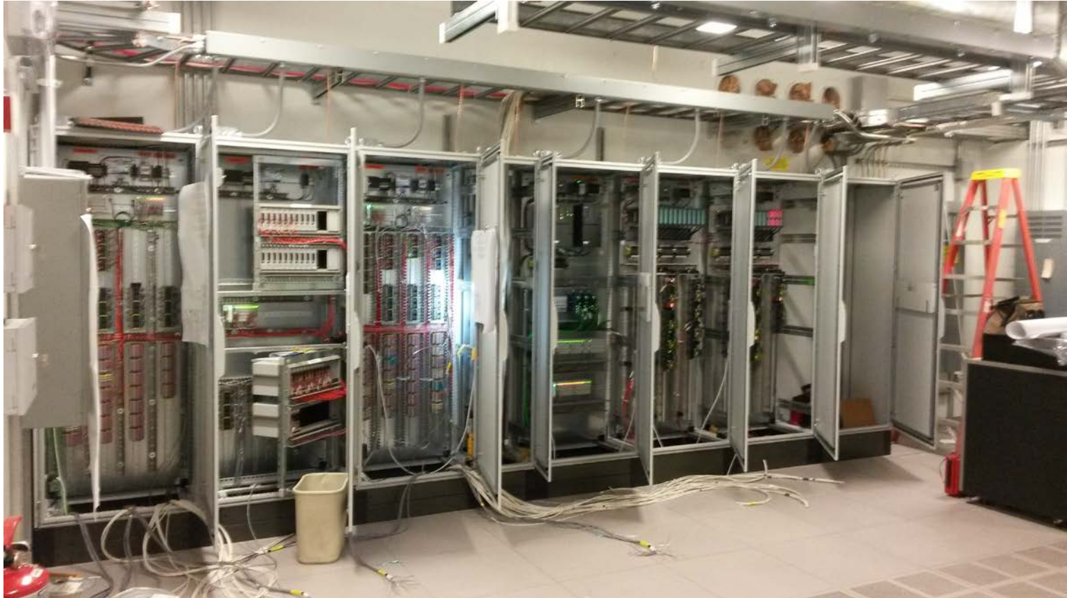
g-2 process controls racks
