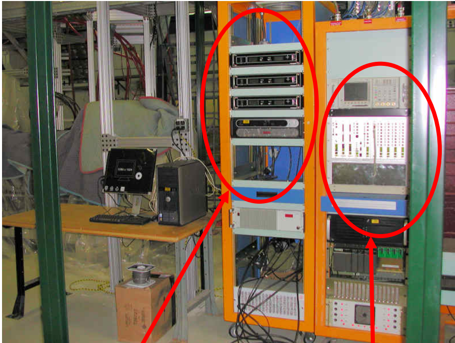
Klystron solenoid power supplies
