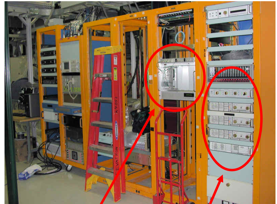
Control system timing crate
