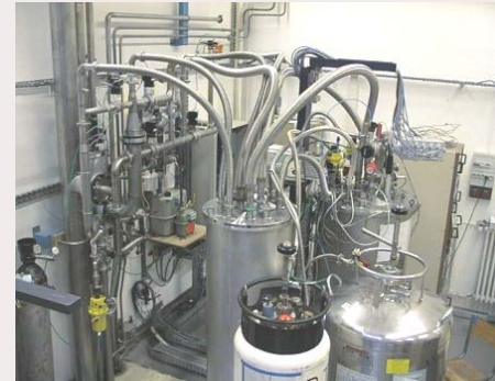
Cryogenic temperature sensor calibration station
