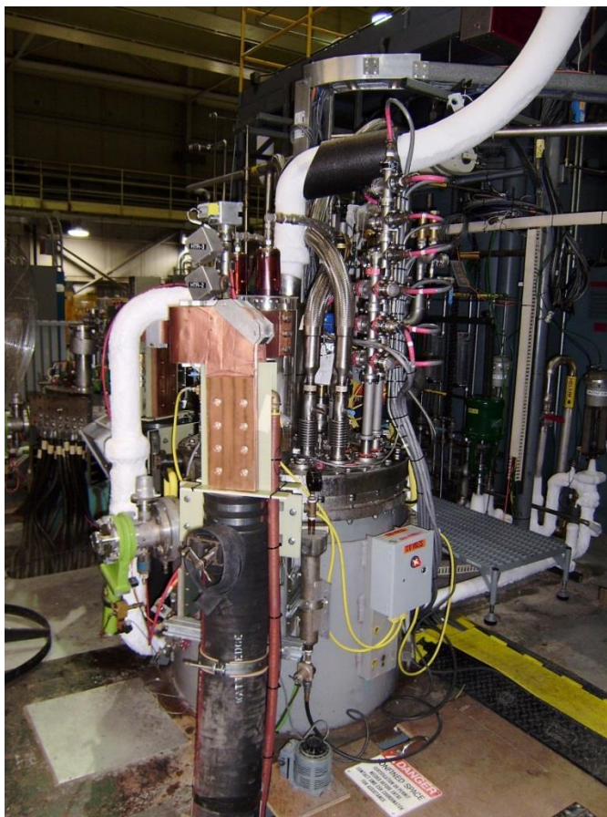
Figure 7.2: Vertical Test Stand 3, upgraded to provide 1.9 K at 1 bar (nom) and 24 kA, for testing of the 4.2 m-long MQXF A quadrupoles. The picture shows the test stand with the mirror MQXFPM1 under test.
