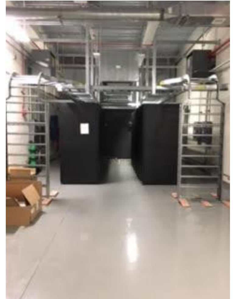
Racks in DAQ Room at Mu2e Hall
