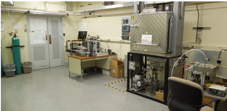
Photocathode Lab – QE measurement, Cathode source material preparation, re-location of vacuum oven
