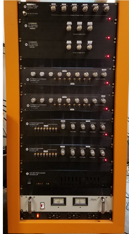
650 MHz LLRF Station for Horizontal Tests
