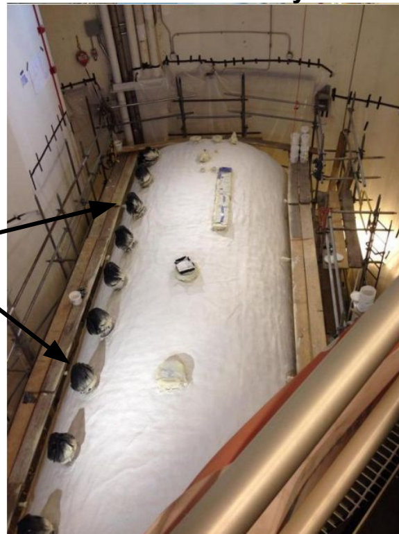
MicroBooNE Foam Insulated Cryostat
