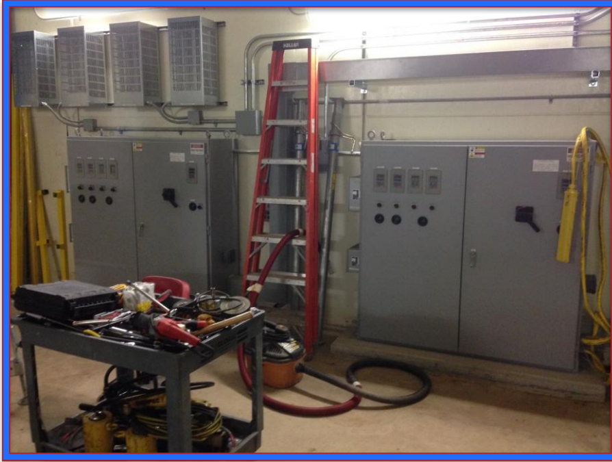
Redundant Crane Controls
