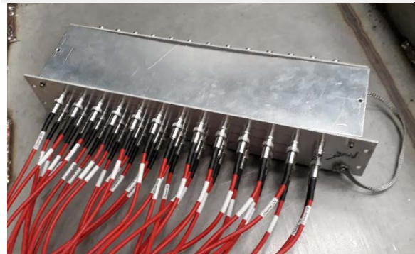
Patch panel to distribute the 14 PS channels to the 42 LEM connexions
