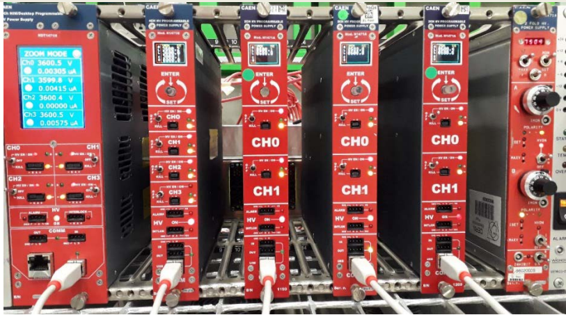
Power supply crate used for the LEMs and grid
