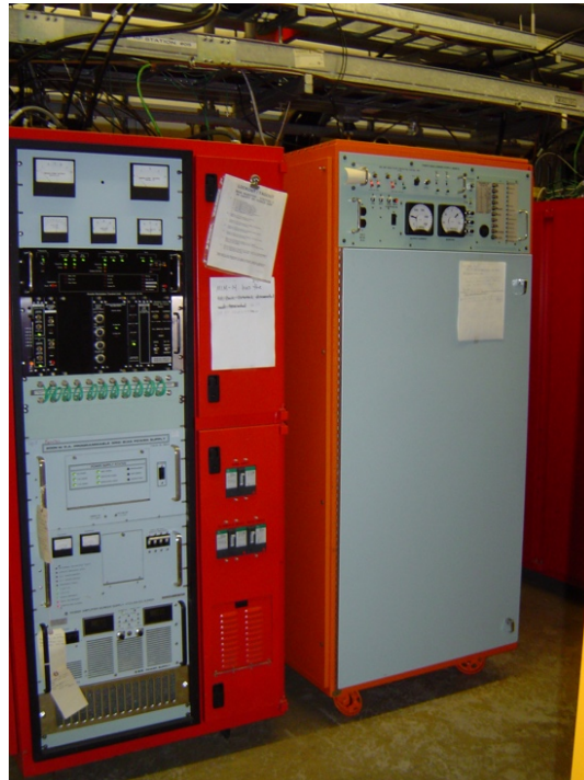
Figure 4.22: Main Injector Modulator (left)
