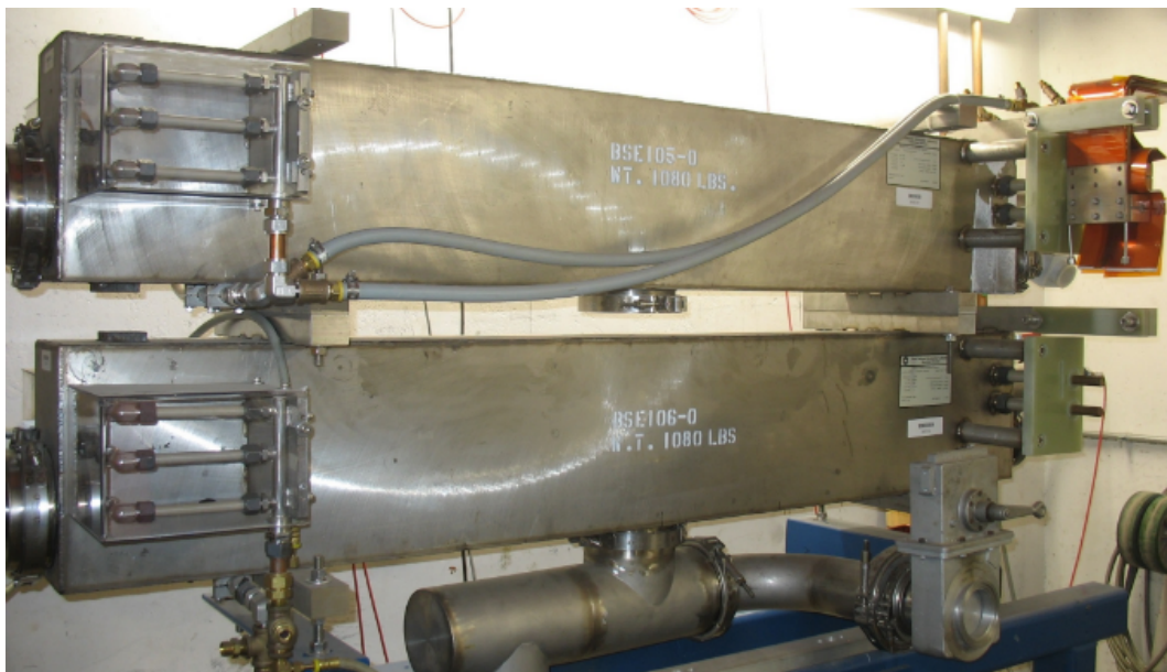
Figure 4.17: Picture of two septa magnets
