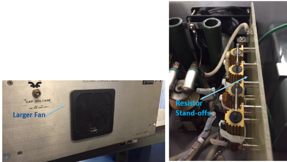
Figure 4.16: Kicker power supply chassis modifications for running at 20 Hz.
