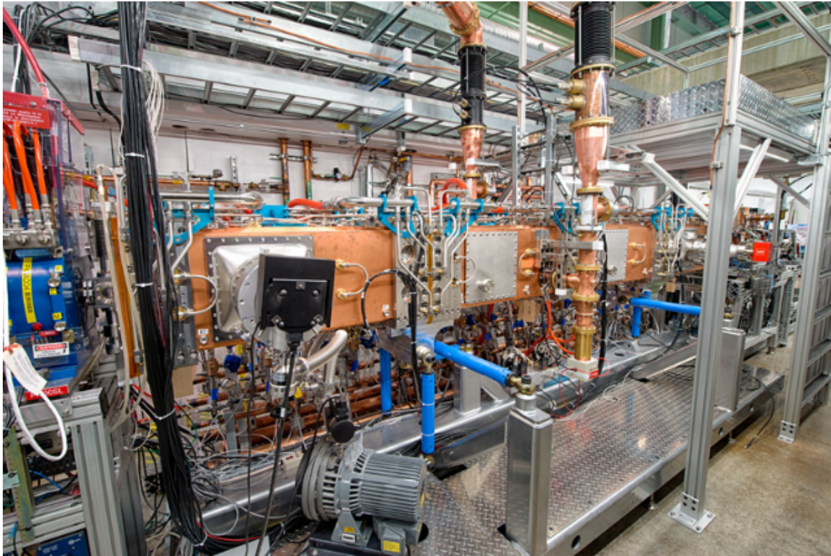
Figure 6.14: RFQ installed in PIP2IT beamline.
