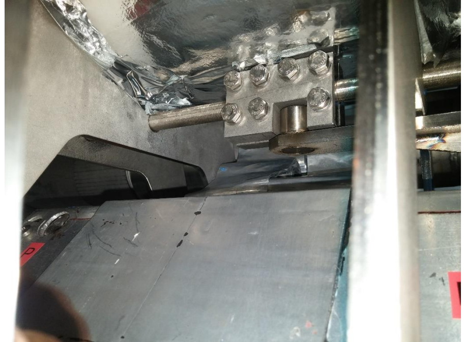
Reinforced clamp design for Cav#1 and Magnet for F1.3-2 & Beyond (to react vacuum forces)
