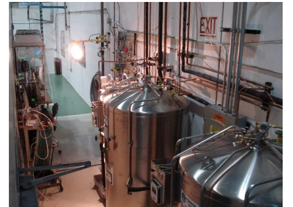
Boiled-off LN2 gas dewars and gas delivery panels
