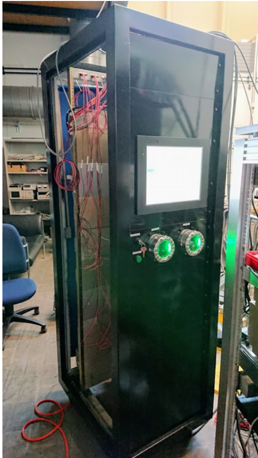
FNAL PLC rack
