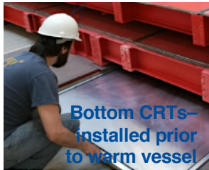
Side CRT East, West, South installation fall 2019
