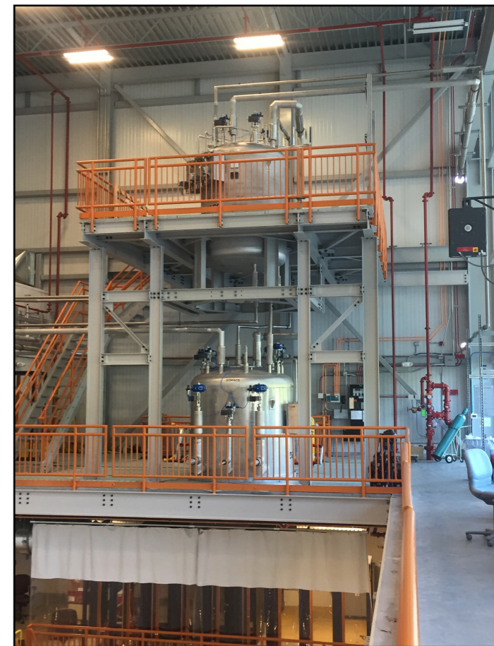
Cryogenic installations in the building
