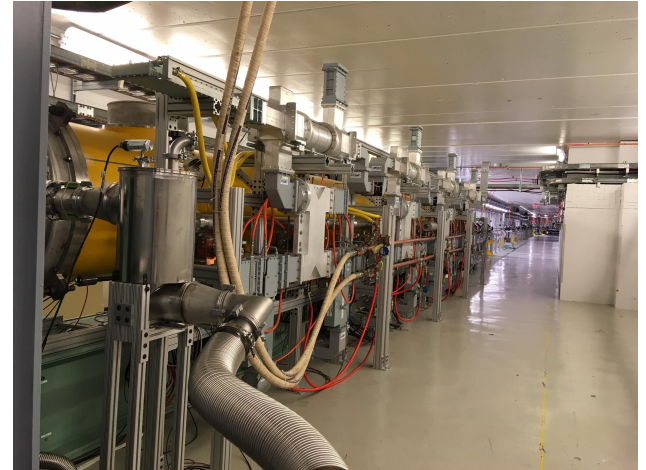
Cryomodule (CM) in linac
