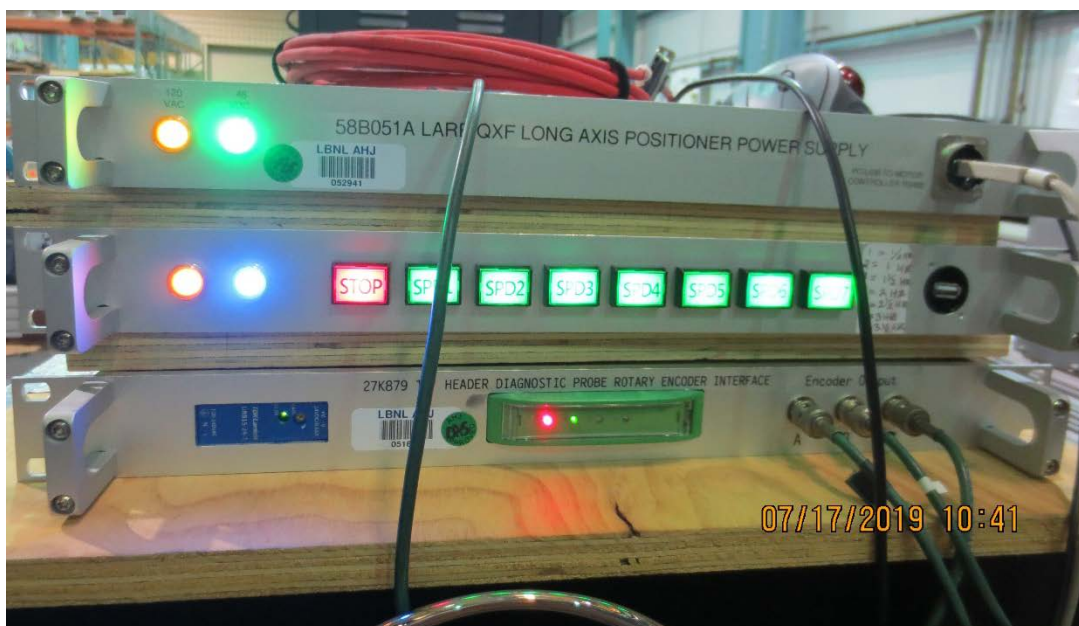
Figure 1: Top Box: power supply & communication to linear motor, Middle Box: speed of rotation control & power supply for rotating motor, Bottom Box: current to voltage converter
