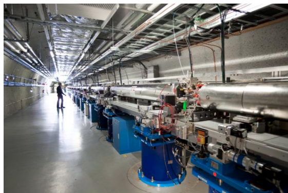
AI is being used to improve modeling and control of particle accelerators systems.
