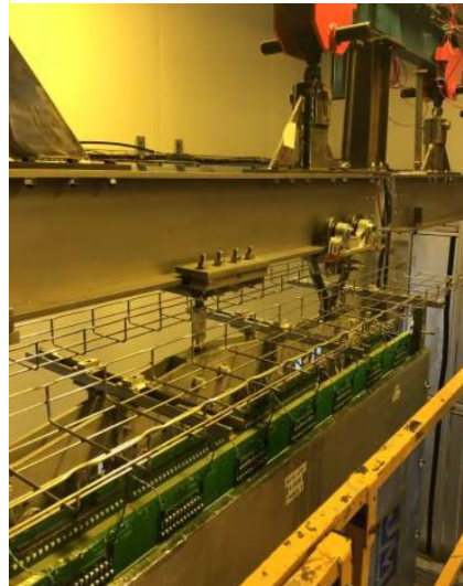
Cable tray installed
