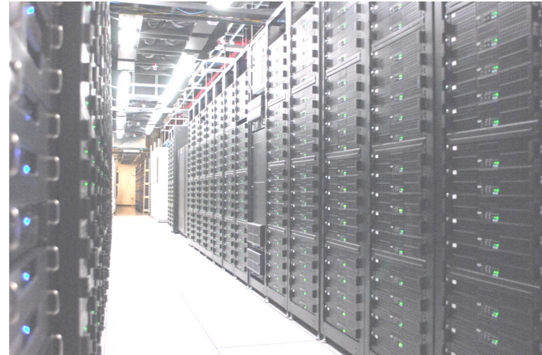
“Kaon” cluster, installed at Fermilab in 2006.
