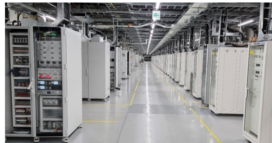
CM/Cryogenic control rack and SSPA
