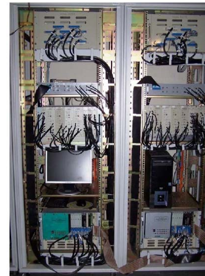
Instrumentation Racks at TIFR
