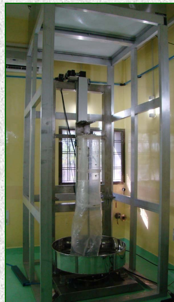
High Pressure Rinsing Set up in Clean enclosure (Class 100)
