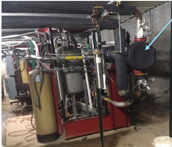
Existing shell and tube HX
