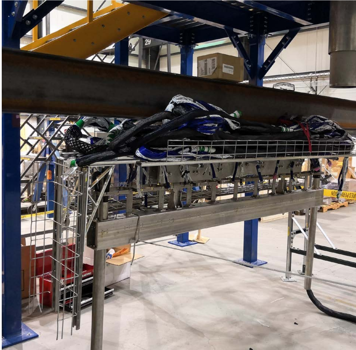
Vertical cable tray installed in the middle
