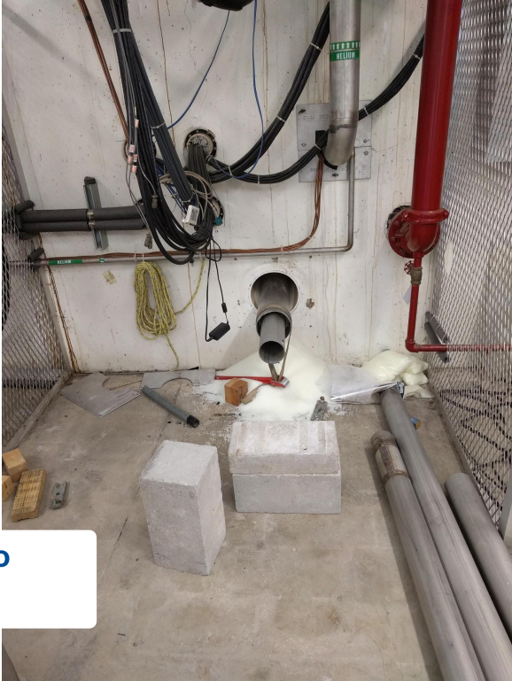
Straight, horizontal penetrations to Counting House room for cryo
