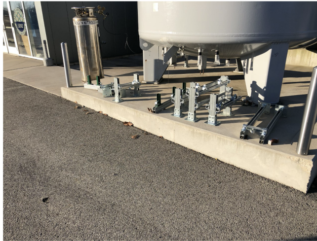
Unistrut support stands outside ND
