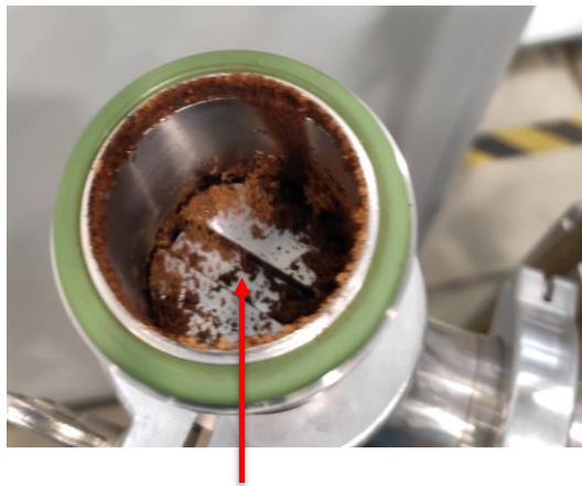
Dirtiness normally observed in the overpressure valve
