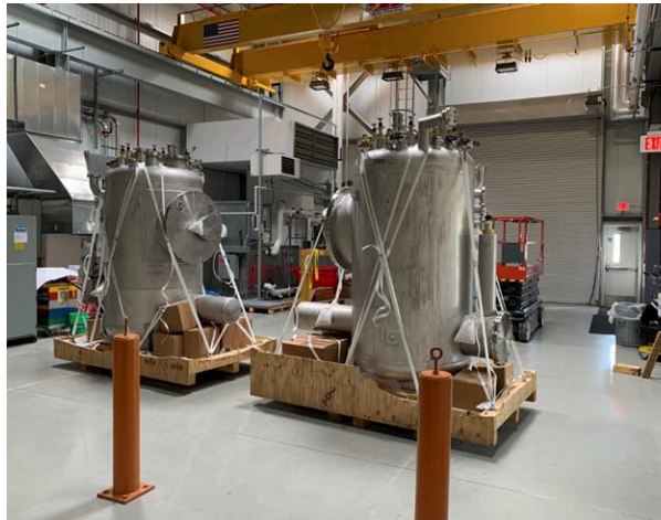
PS and DS cryo distribution boxes
