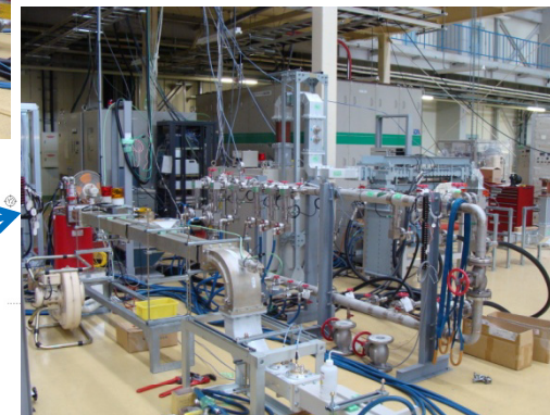
30 kW klystron and IOT
